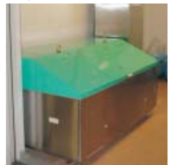
Garbage disposer installed at Nagasaki Branch Office
