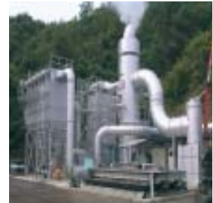
Incineration unit using a dioxin removal system
