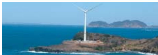
Kushizaki Wind Power Station in Chinzei Town, Higashi-matsuura-gun, Saga Pref. (1,980 kW, subsidized in FY2003)
