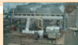
Binary cycle power generation facilities
