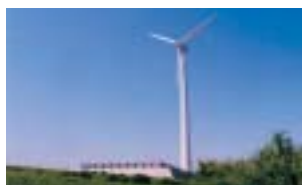
Wind-generated power equipment located in Itsuwa Town, Kumamoto
