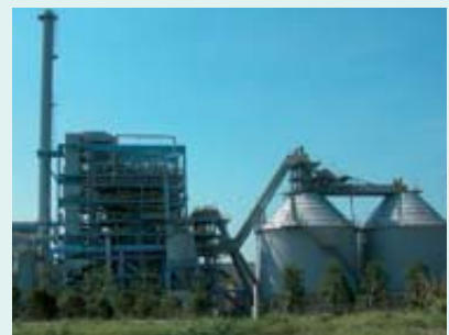
The Miyazaki Biomass Recycling Power Station
