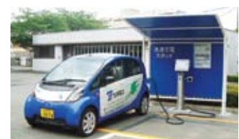
Electric vehicle at a rapid recharging stand
