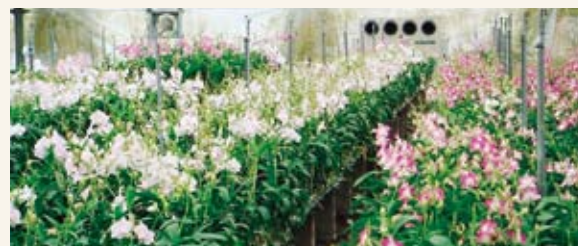
Heat pump in orchid greenhouse
