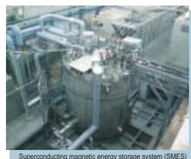
Superconducting magnetic energy storage system (SMES)
