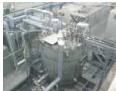
Superconducting magnetic energy storage system (SMES)
