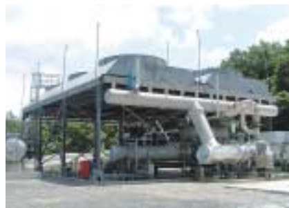
Hatchobaru Binary Cycle Power Plant
