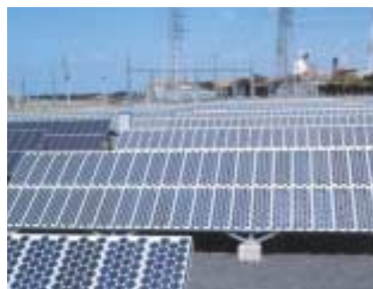
Photovoltaic power generation equipment at Karita Power Station
